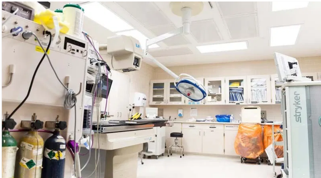
LED lighting at Russell Medical Center, which has benefitted from the new lighting installed by Energy Focus. Photo Credit: Energy Focus
